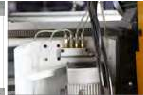
YAĞLAMA SİSTEMİ LUBRICATION SYSTEM
